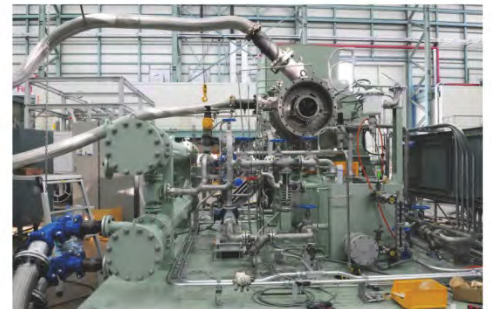
Combined Cycle Power Plant
