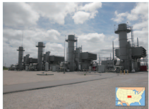
Fig. 4 LM6000x4 Emporia Power Station
