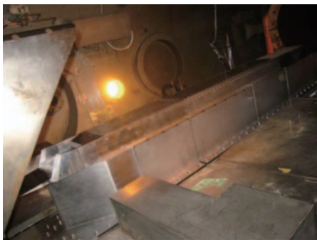
Fig.14 The S-engine installed in the ramjet engine test facility (8)
