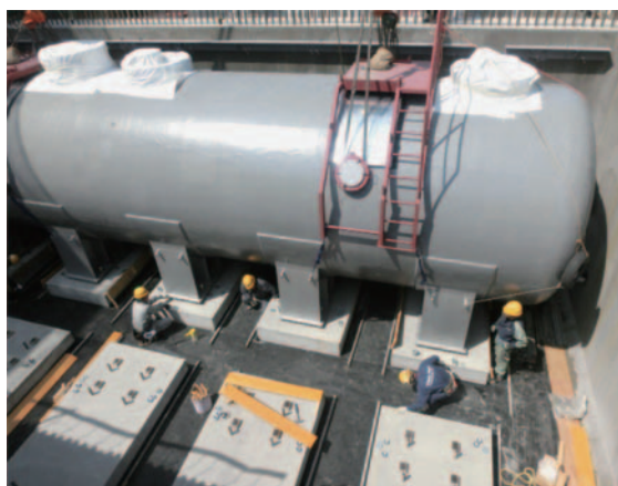
Fig. 6 The fuel tank under the ground.
