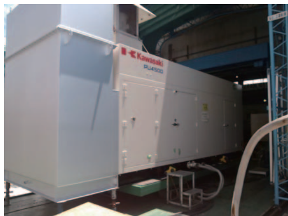
Fig. 3 Dual Fuel Gas Turbine Generator
