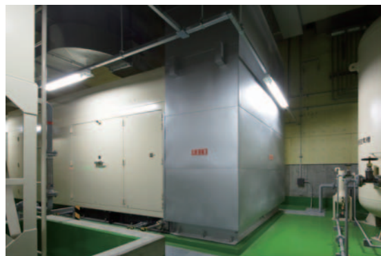
Fig. 4 Dual Fuel Gas Turbine Generator
