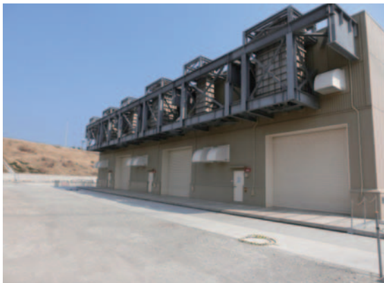
Fig. 2 The seismic isolated building in which the gas turbine generators are installed.
