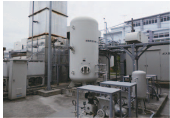
Fig. 2 Starting Air Compressor
