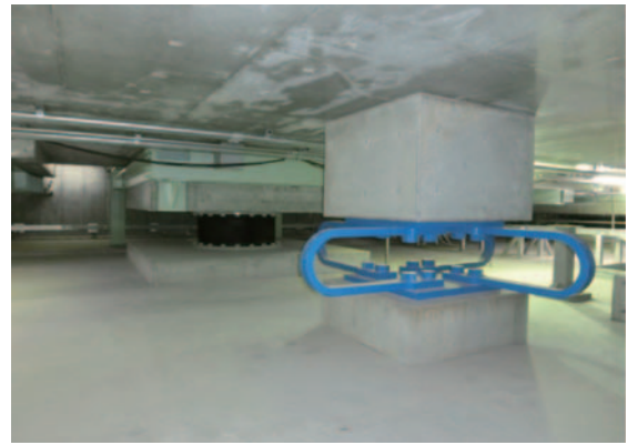
Fig. 3 The seismic isolation systems at the basement of the building.
