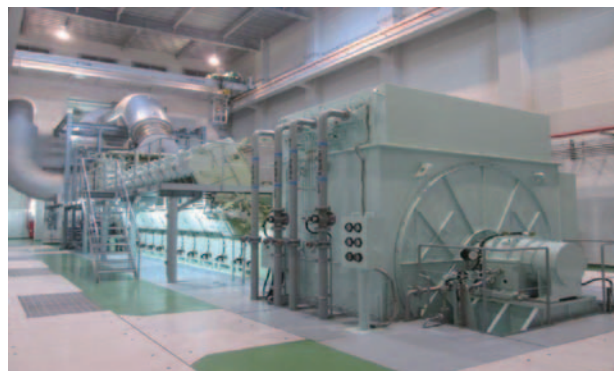
Fig. 4 Ishigaki No.2 power plant (diesel generator)
