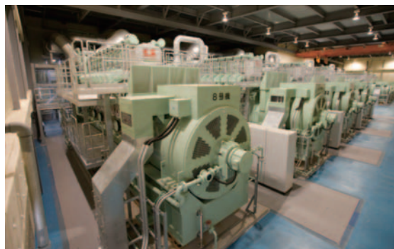
Fig. 2 Inside of Sodegaura Green Power Plant
