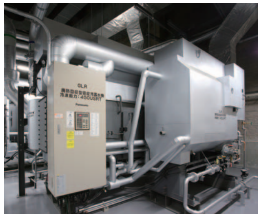
Fig. 7 Heat recovery absorption chiller (Hot water utilization)
