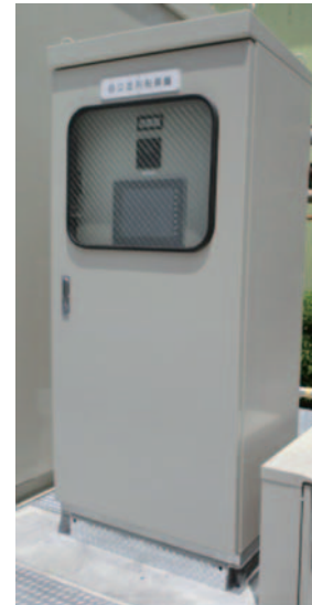
Fig. 10 Control panel for load sharing
