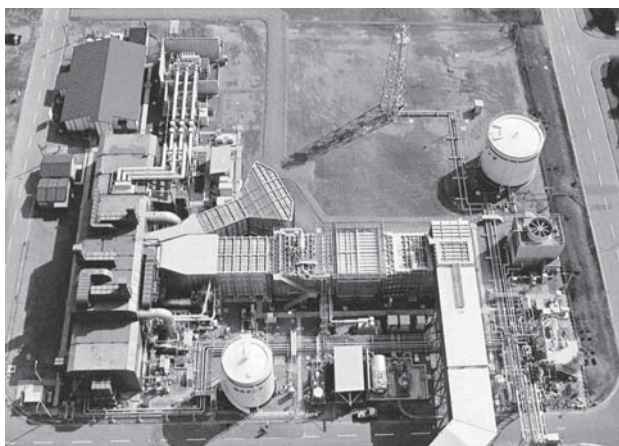
Fig. 3 The pilot plant under trial operation (Sodegaura thermal power plant of Tokyo Electric Power Company)
