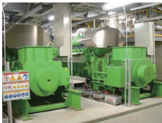
Fig. 10 Gas engine and generator
