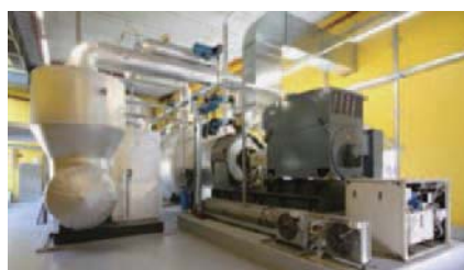
Fig. 9 ORC unit for biomass plant
