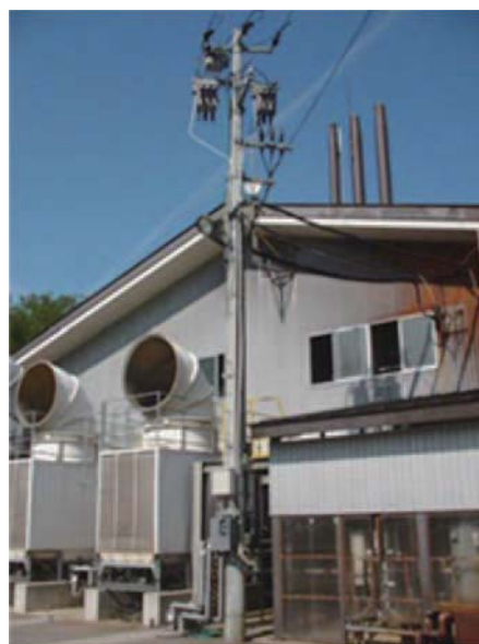
Fig. 11 Electric power transmission equipment
