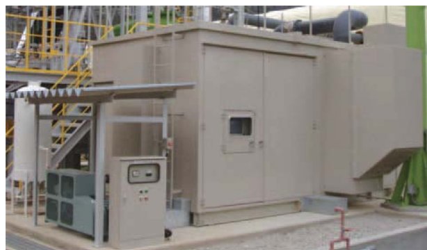
Fig. 13 External view of gas-turbine package
