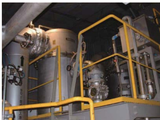
Fig. 9 Gas cleaning equipment
