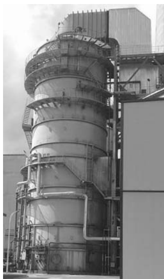
Fig. 7 Limestone-gypsum desulfurization unit
