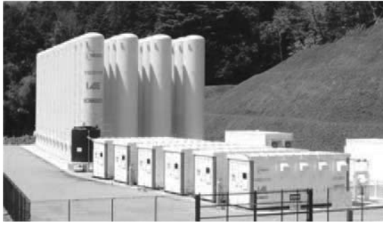
Fig. 8 Outer view of the CAES test facility
