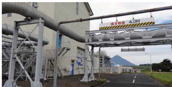
Fig. 9 Yamagawa Geothermal Power Station
