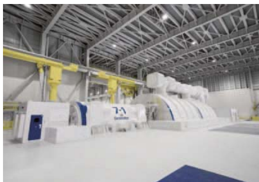
Fig. 7 TC4F-48" Steam Turbine and Generator
