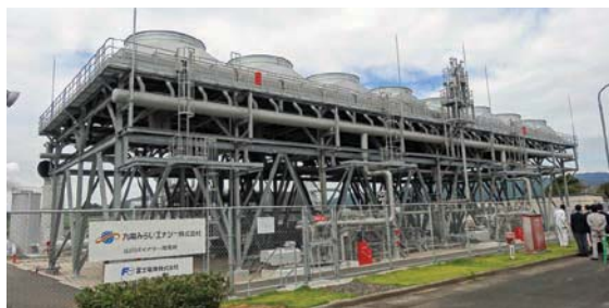
Fig. 10 Yamagawa Binary Power Station
