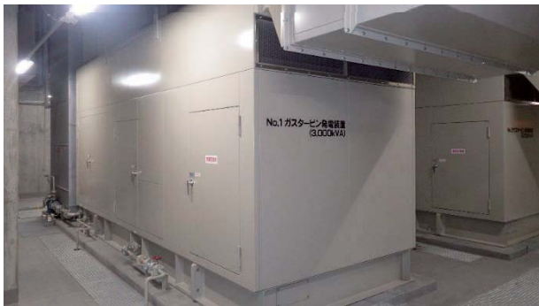
Fig. 2 Emergency power generation system
