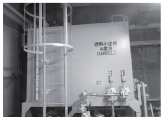
Fig. 3 Fuel small tank
