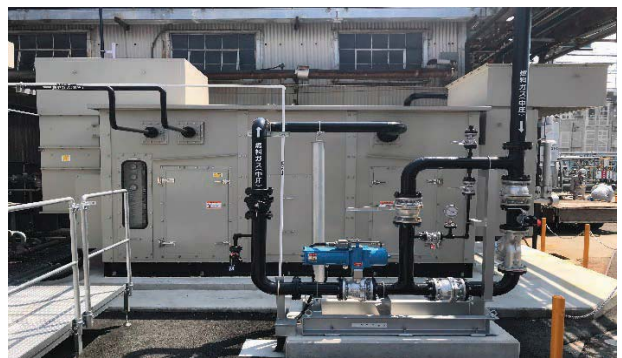
Fig. 6 Air-cooled gas compressor package
