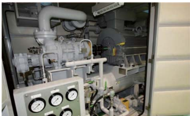
Fig. 2 Gas compressor unit (model 160M)
