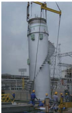
Fig. 18 Sample of Exhaust Stack
