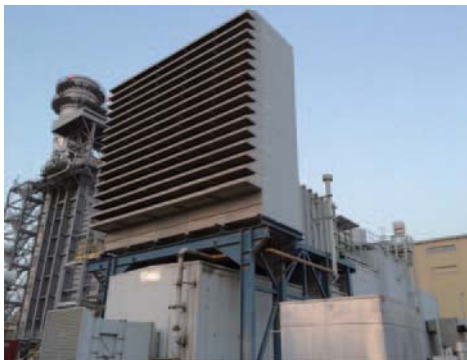
Fig. 8 Sample appearance of GT air intake filter house which contains Cartridge type filter
