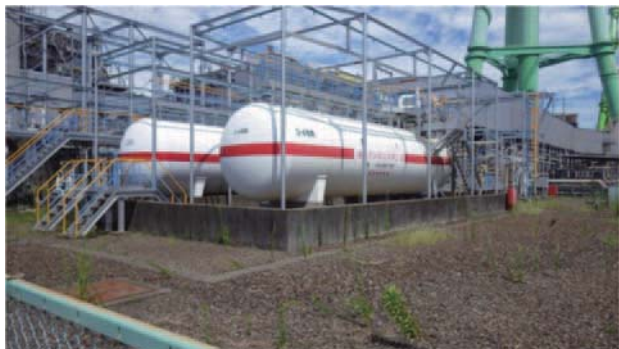
Fig. 4 Ammonia supply facility
