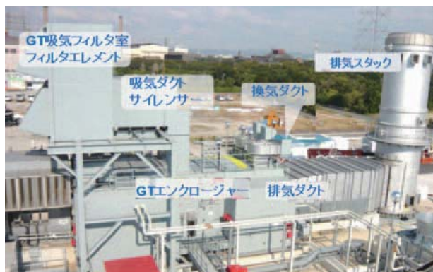
Fig. 10 Sample appearance of the whole GT package and our handled equipment
