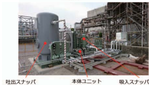
Fig. 5 Ammonia gas compressor
