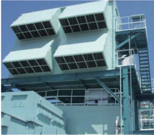
Fig. 11 Sample of GT intake filter house (1)
