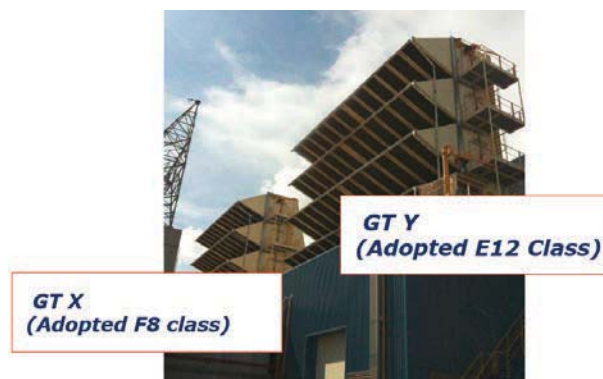
Fig. 1 GT intake filter house
