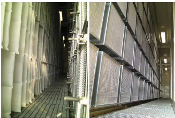
Fig. 3 HEPA filters in GT intake air filter house
