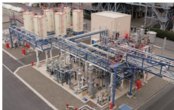
Fig. 12 Dehydrogenation plant (Kawasaki city)
