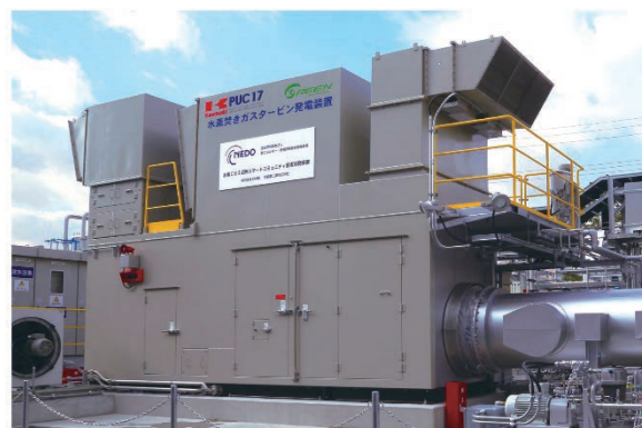
Fig. 7 Hydrogen CGS demonstration plant
