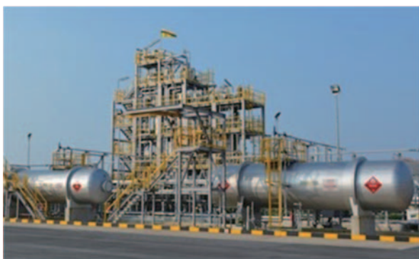
Fig. 9 Hydrogenation plant (Brunei darussalam)
