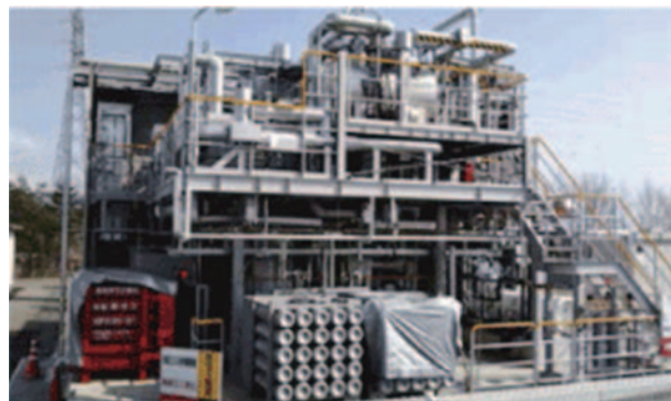
Fig. 3 Ammonia synthesis demonstration plant
