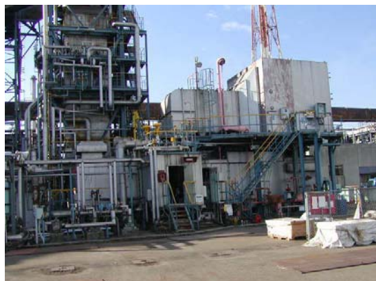
Fig.7 Nippon Petroleum Refining Co., Ltd. Mizushima Refinery
