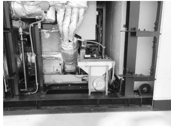
Fig. 13 MGT installed in SOFC
