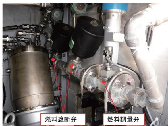
Fig. 2 Ammonia supply unit in the package
