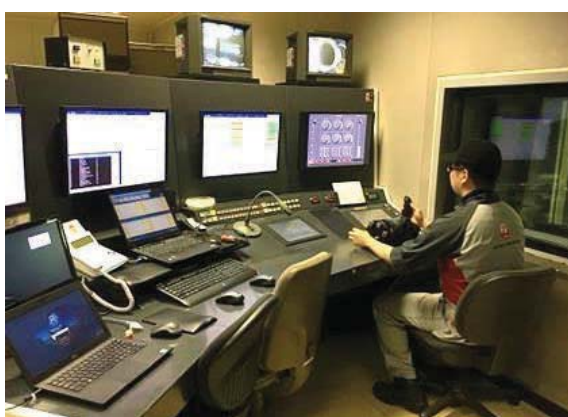
Fig. 4 Engine Control Panel
