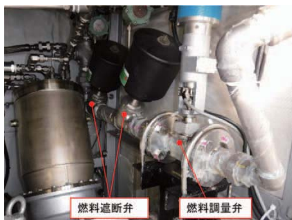
Fig. 2 Ammonia supply unit in the package
