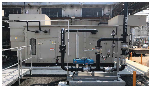
Fig. 6 Air-cooled gas compressor package
