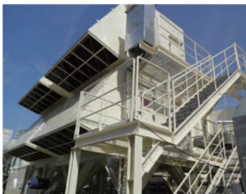
Fig. 12 Sample of GT intake filter house (2)
