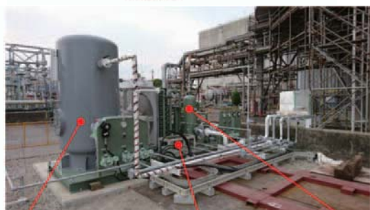
Fig. 5 Ammonia gas compressor
