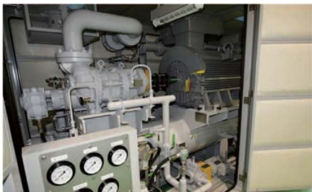
Fig. 2 Gas compressor unit (model 160M)
