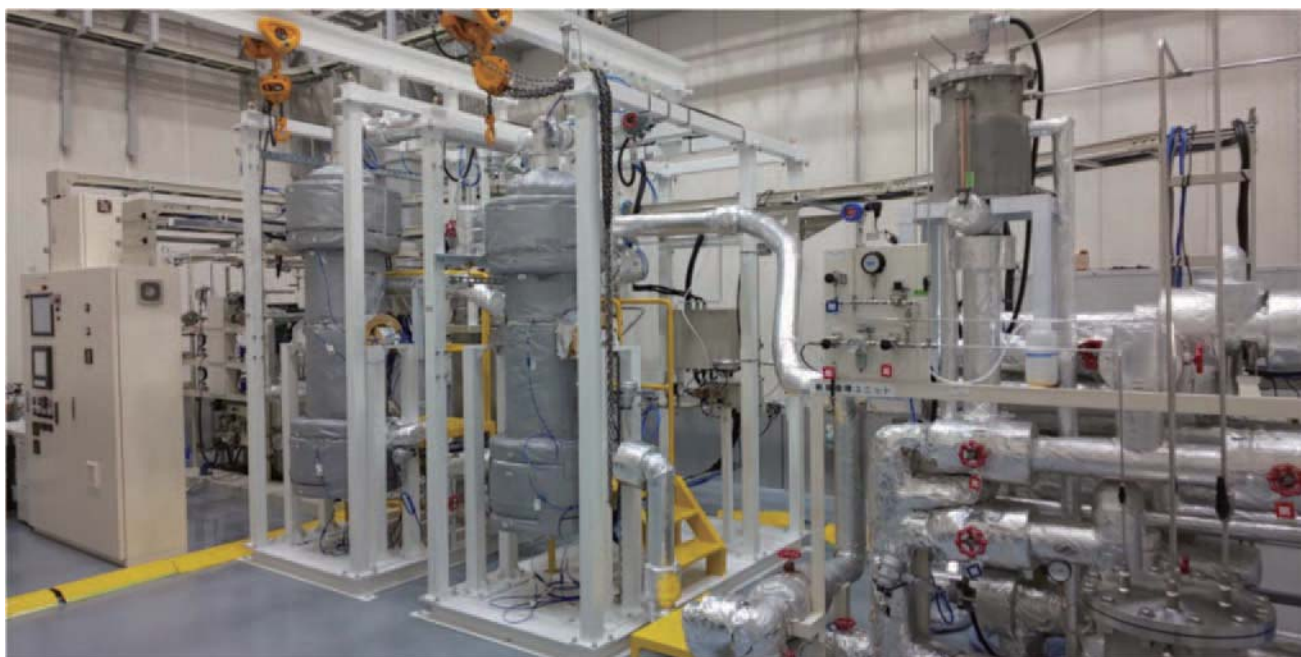
Fig. 10 Methanation bench test facilities
