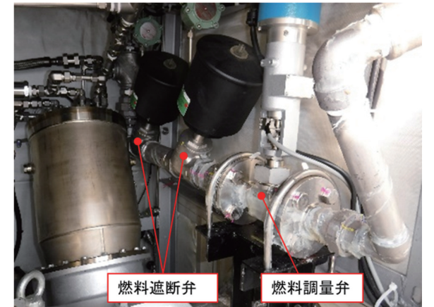
Fig. 2 Ammonia supply unit in the package
