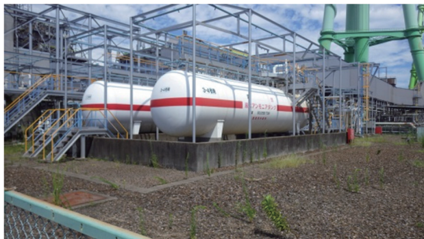
Fig. 4 Ammonia supply facility
